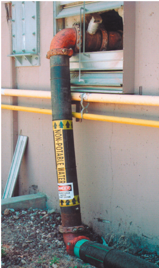
The temporary, above ground pipe stretches a quarter mile (400 m) from the city's treatment plant to the mill
